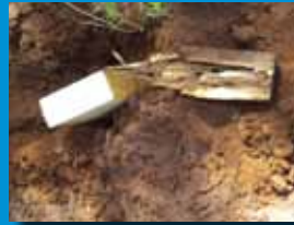
Treated and untreated wood damage
